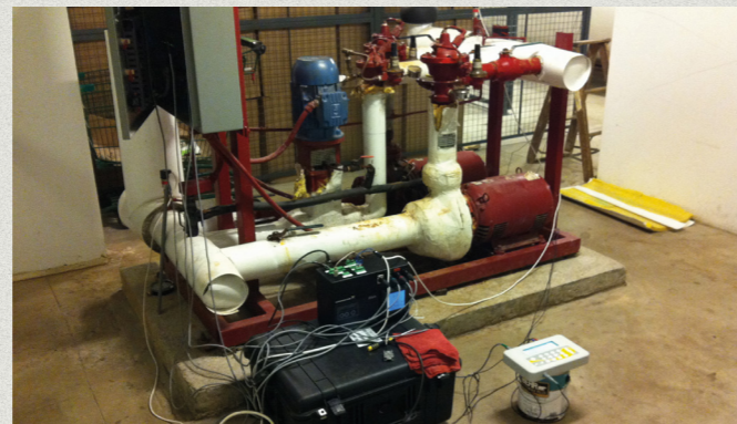
Pump monitoring equipment in use
