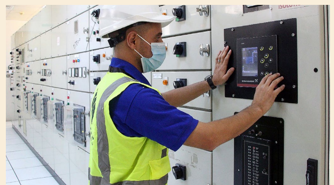
With dedicated controls and a remote management system from Grundfos, RAKWA saved 20% energy and 12% in total operational costs with a pump system upgrade on its wastewater system.
