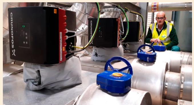
George Nicholls, Arla Foods, and the new TPE pumps for the ice water system
