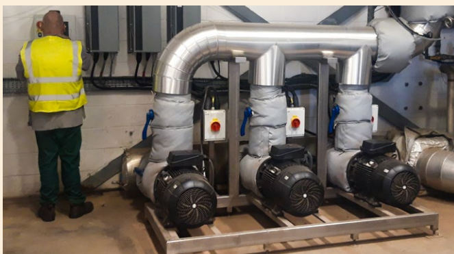
The new chilled water NB pumps
