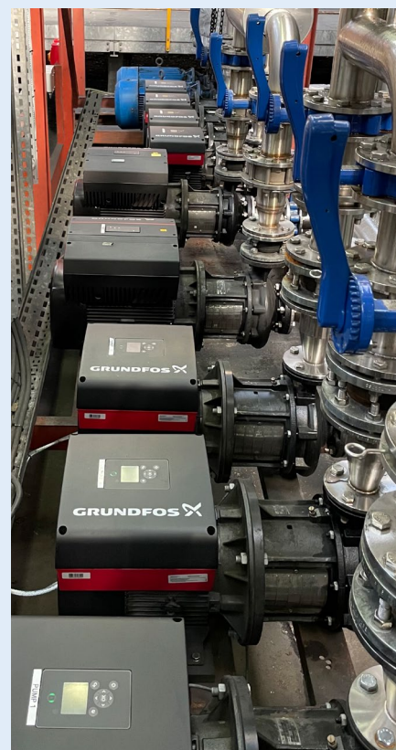
Grundfos NBE pumps for Suntory Beverage & Food's chilled water system.
