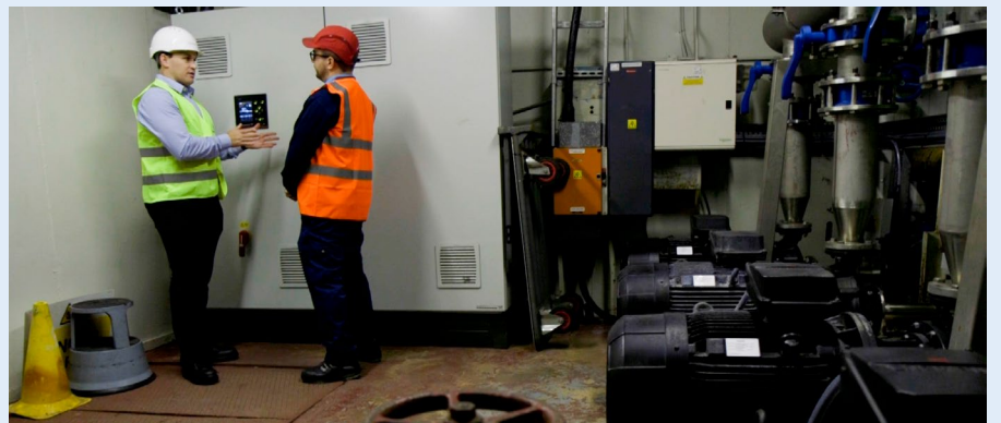
The town's water facility at Suntory Beverage & Food's GB&I factory
