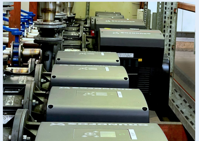
A series of 14 dual pump Grundfos NBE systems with 11 kW premium-efficient IE5 motors run on constant pressure control for Lucozade's Central Chilled application.
