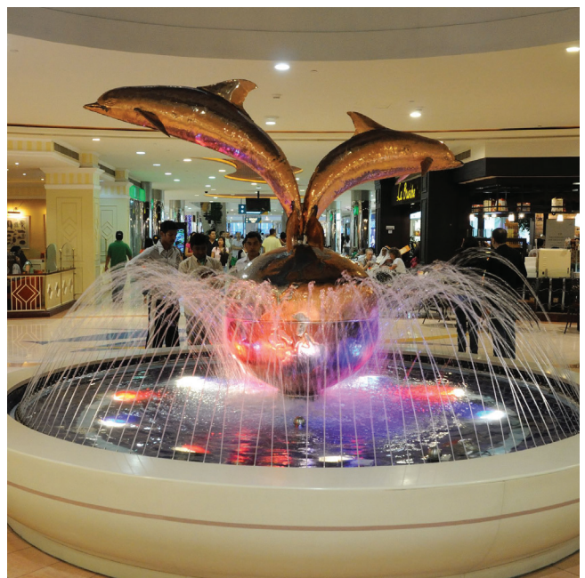
Water fountain in a shopping mall.
