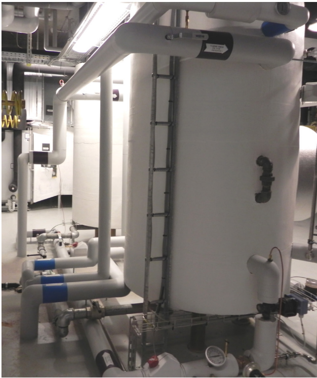
Insulated hot water tanks in a commercial building.
