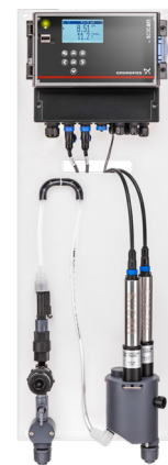
Figure 2: Measurement and control systems are used to determine the residual level in the water at a specific sampling point.
