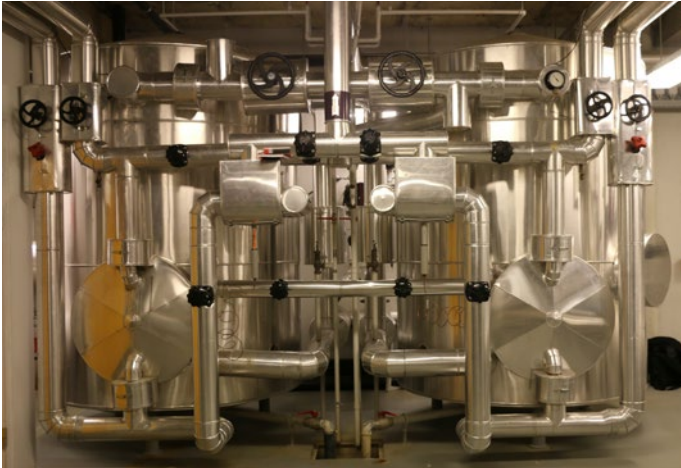
One of the two hot water preparation plants at the regional hospital of Viborg
